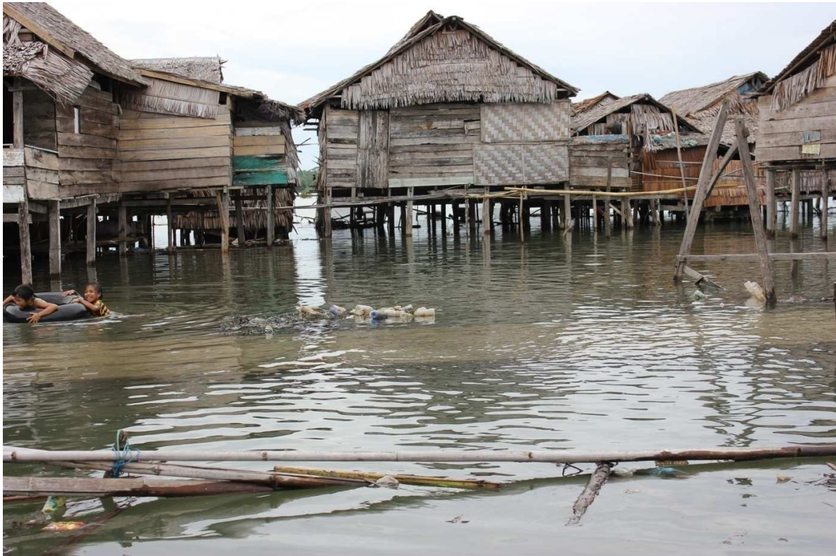
Figure 16: Local house condition at high tide in Ulo-ulo sub-district, Luwu district (Photo by Ikhsan, 2011)
